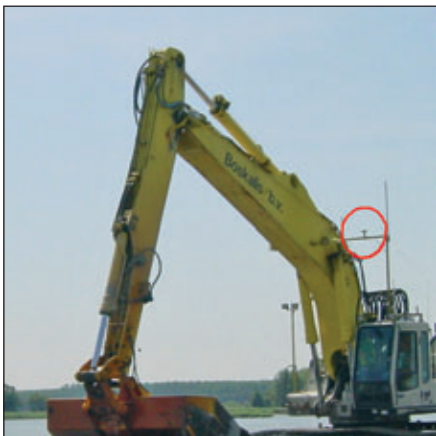
Installation on a dredging vessel. A location on top of the cabin is chosen.
