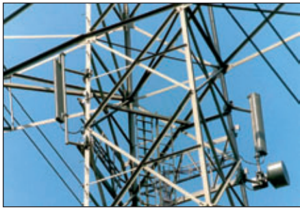
Figure 4: GPS is not only used for positioning, but also for switching power and telecommunications. (source: www.convvoj.ch )
